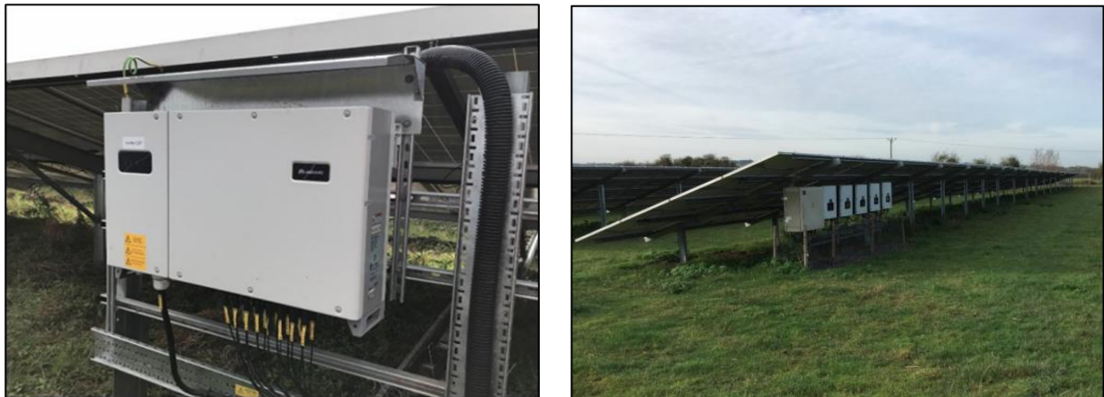
Plate 3.3 Typical String Inverter
